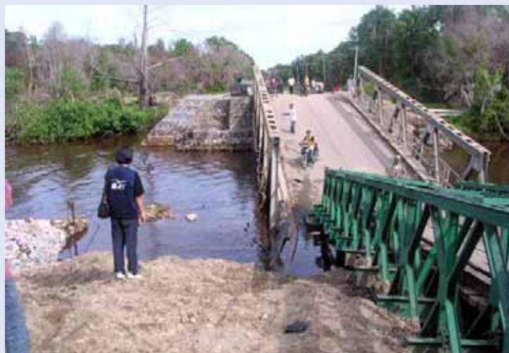
Dewi, a JRS volunteer, and the collapsed bridge in Tapaktuan
